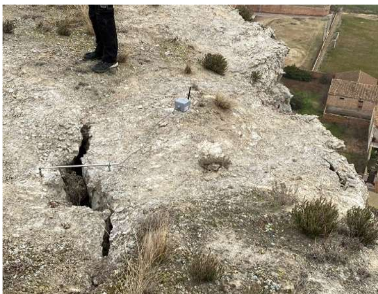
Crack meter installed across the crack on the rock
