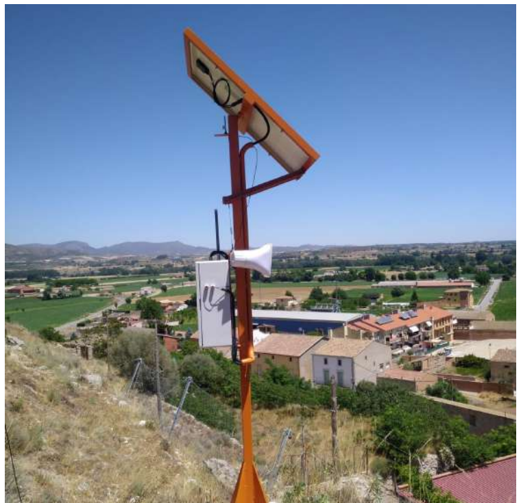
The alarm and siren system installed on the cliff
