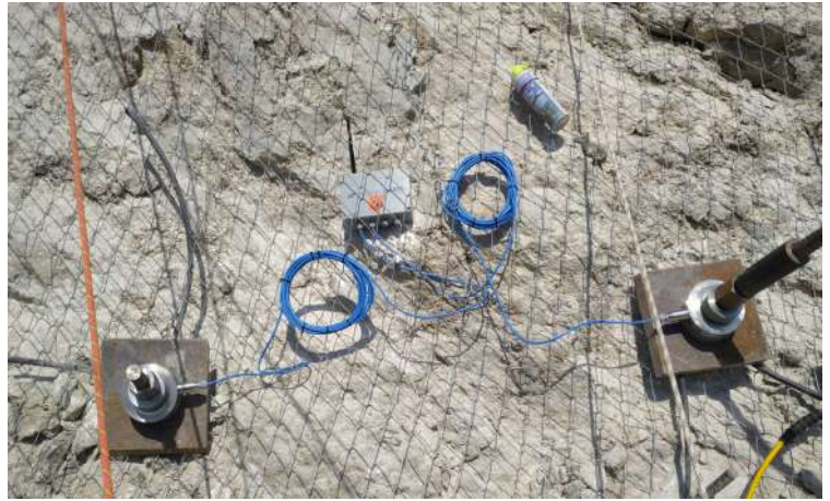
Load cells installed with RF datalogger on the rock bolts installed for the rock stabilization
