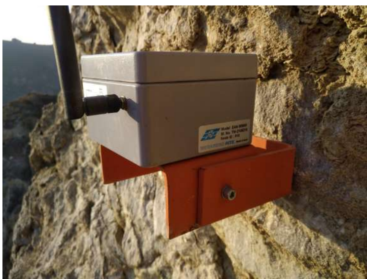
Wireless tilt meter with in-built RF datalogger, installed on the rock
